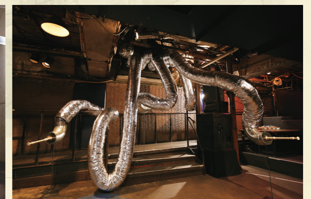
work with #9 (CLUB METRO 空調設備)
